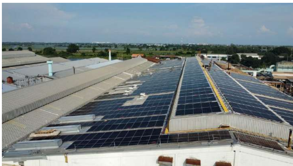
Project of Solar rooftop
